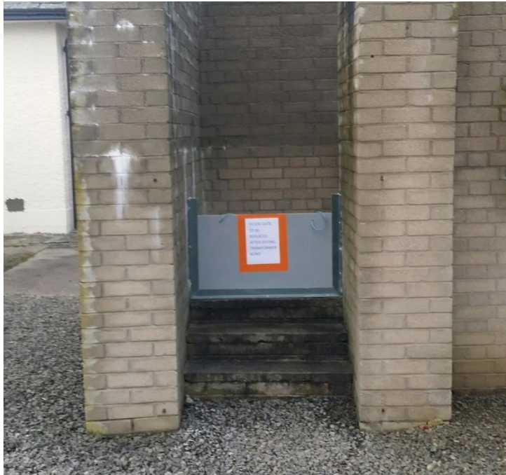
Photograph 6 – Example of a grid substation switchroom access with additional flood gate protection
