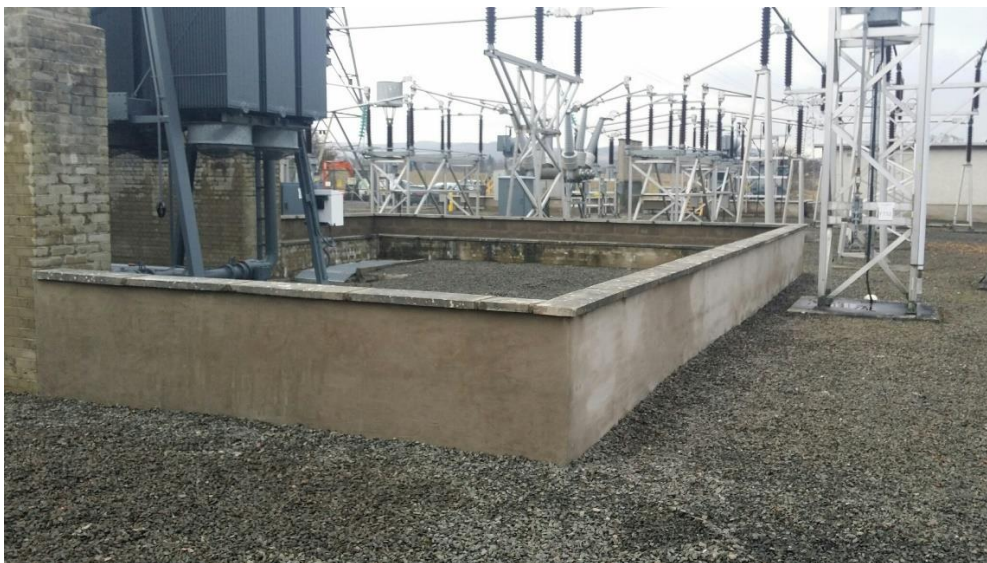
Photograph 4 & 5 – Example of a HV transformer and associated control equipment protected by a raised bund wall with step access
