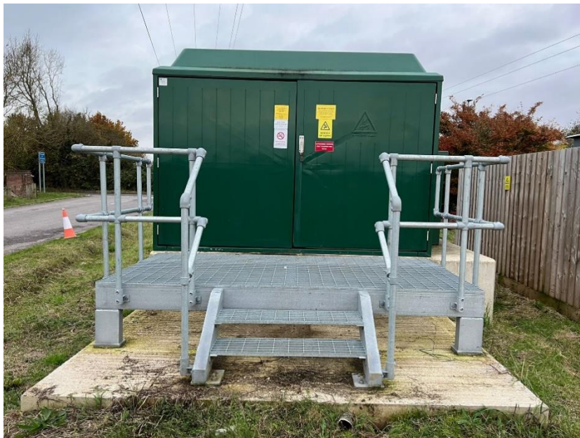
Photographs 1 & 2 – Example of enhanced flooding protection
