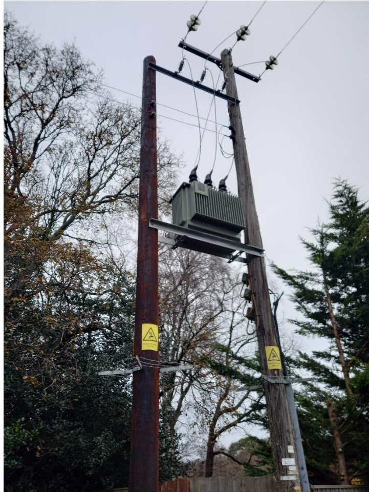
Photograph 3 – Example of a pole mounted transformer with surge arresters
