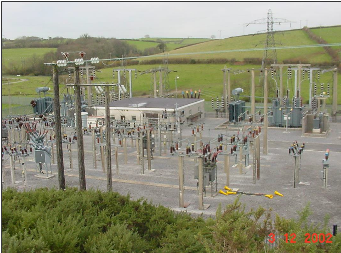
Photograph 5 - 132kV Grid Substation showing 132kV terminal tower (pylon) and start of 33kV wood pole overhead line
