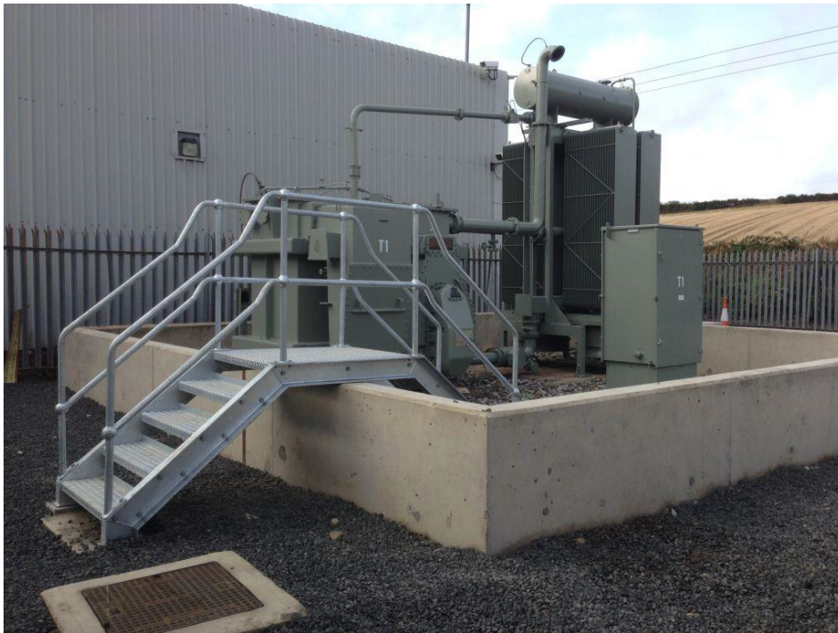
High voltage transformer and associated control equipment protected by a bund wall with step access. (Courtesy NIE)
