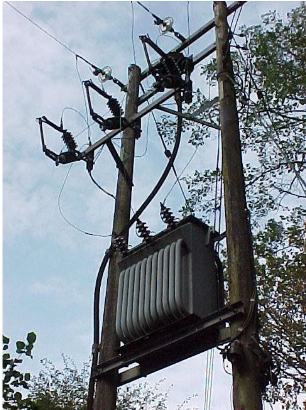
A pole mounted distribution transformer with external cooling tubes.
