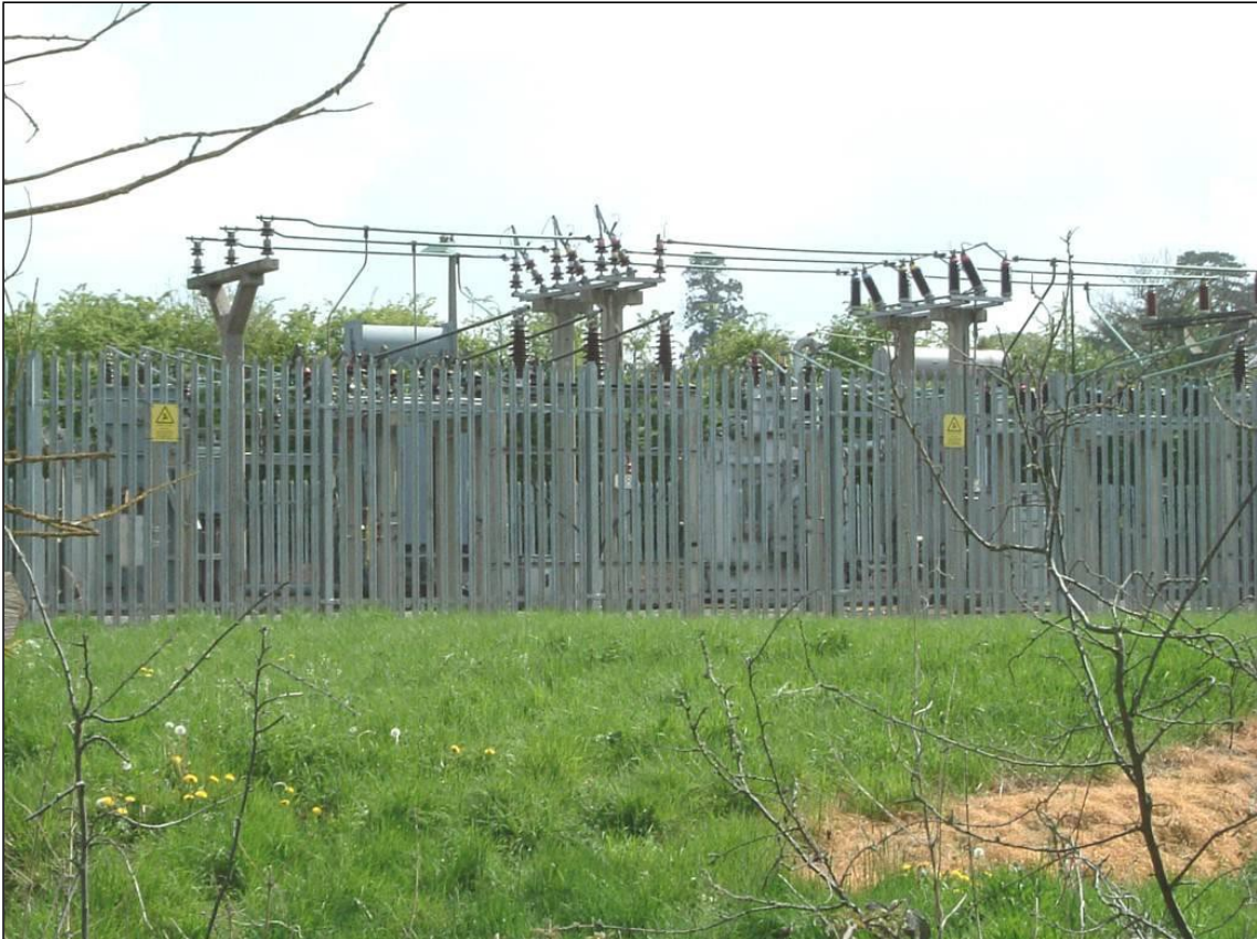
Photograph 6 - Primary Substation showing equipment operating at 33kV and 11k
