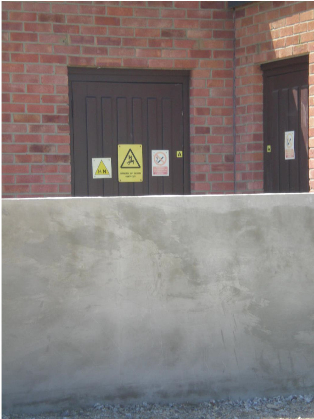
Flood defence wall – designed to allow access into the substation during a flood – SSEPD.
