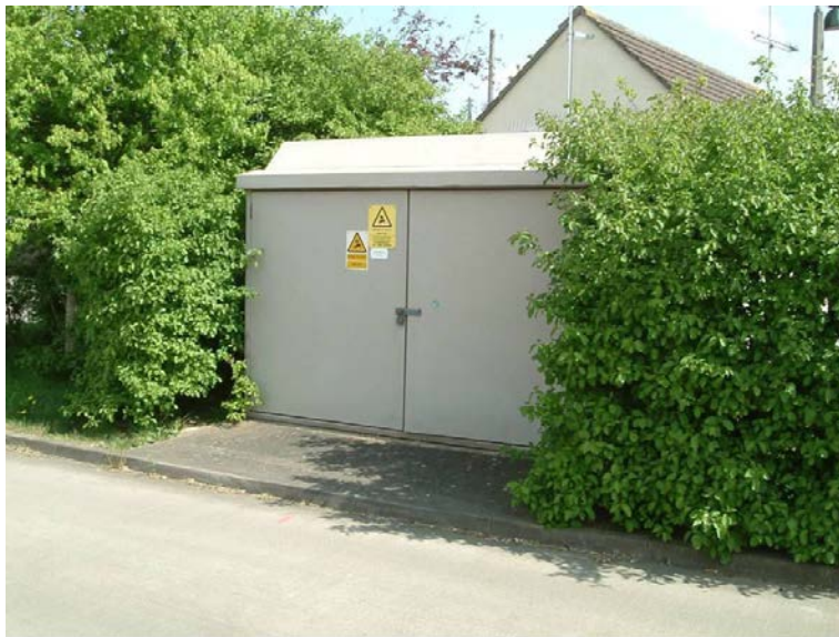
Distribution Substation with equipment operating at 11kV and 400/230 volts
