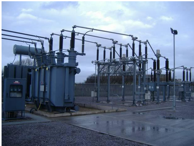
132kV Grid Substation showing main power conductors at high level but control circuits located in cubicles at lower level
