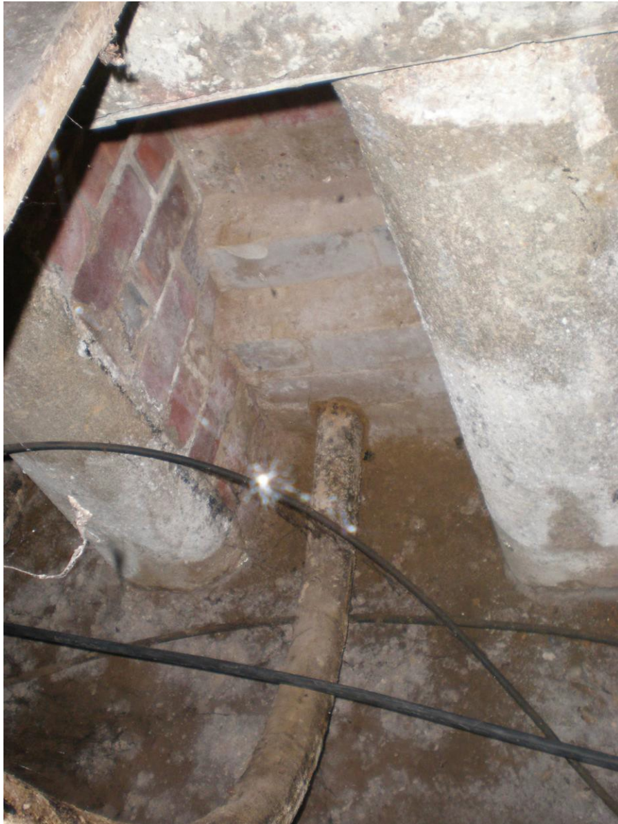
Example of cable sealing - SSEPD
