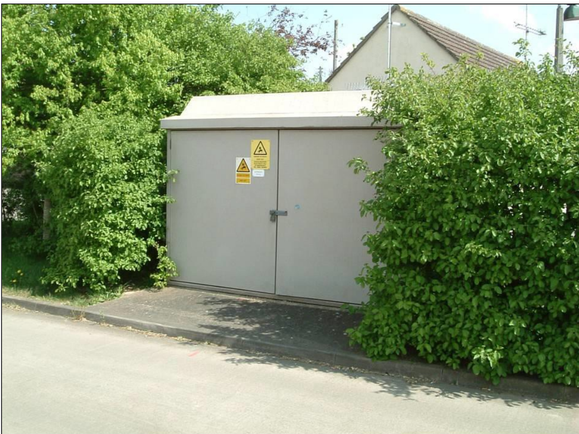
Photograph 7 - Distribution Substation with equipment operating at 11kV and 400/230 volts
