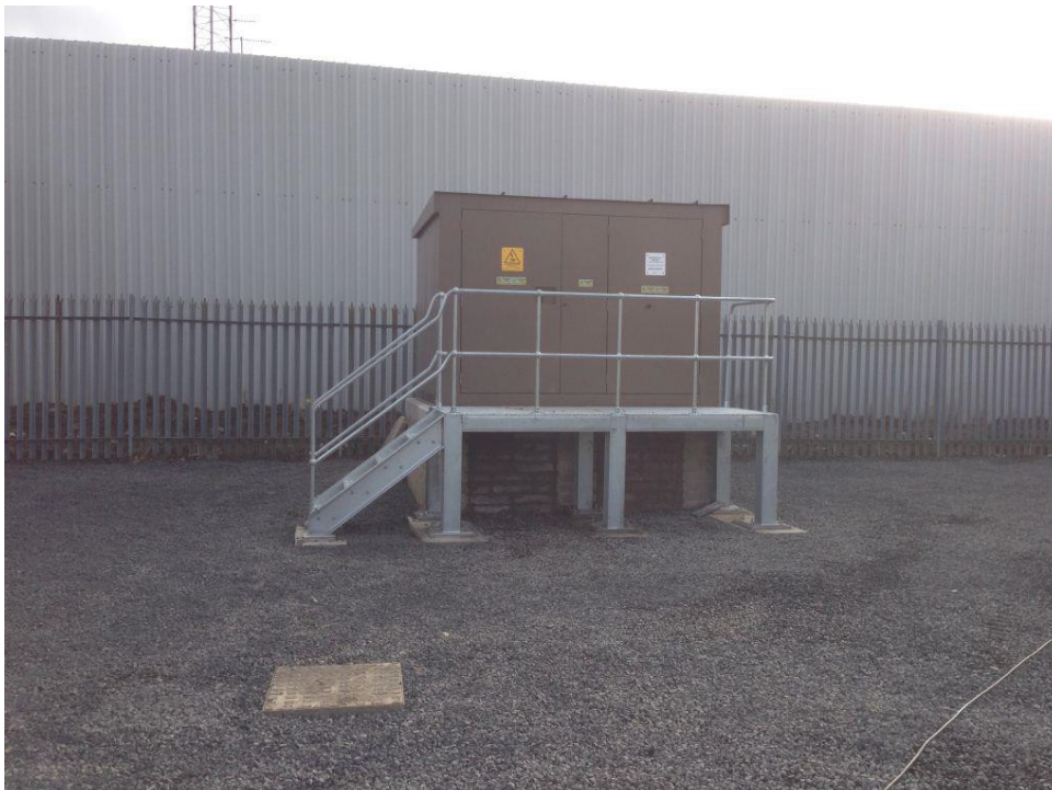
Control equipment protected on a raised plinth with step access. (Courtesy NIE)
