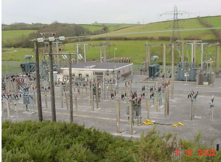
132kV Grid Substation showing 132kV terminal tower (pylon) and start of 33kV wood pole overhead line.
